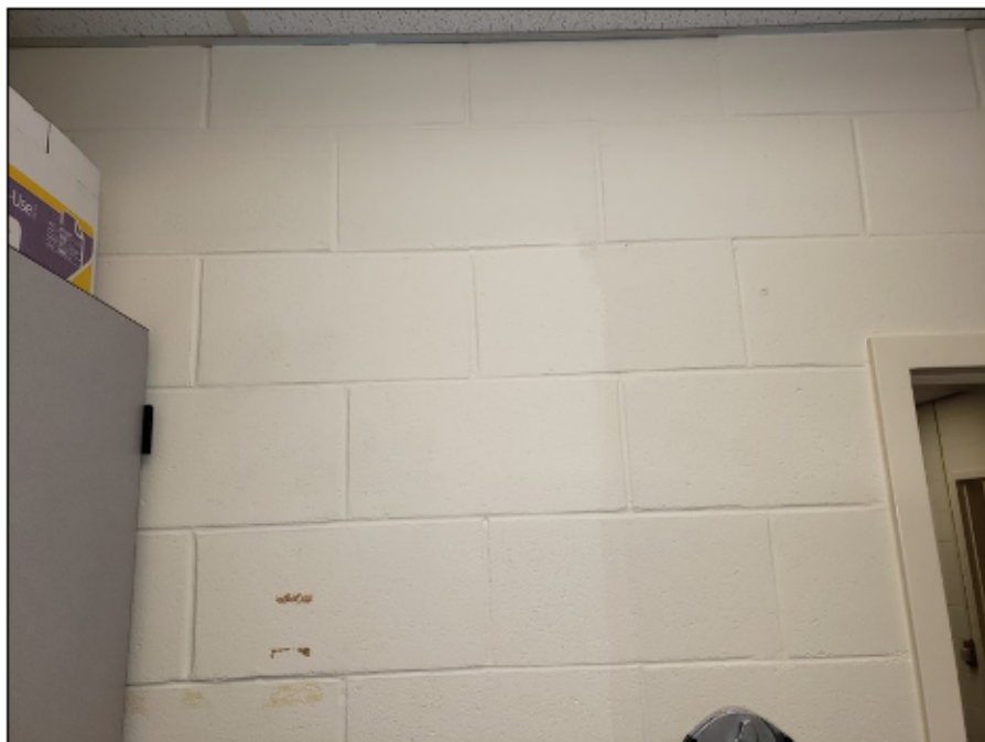
1 - Trace <1% Asbestos - CMU Block Filler Paint
