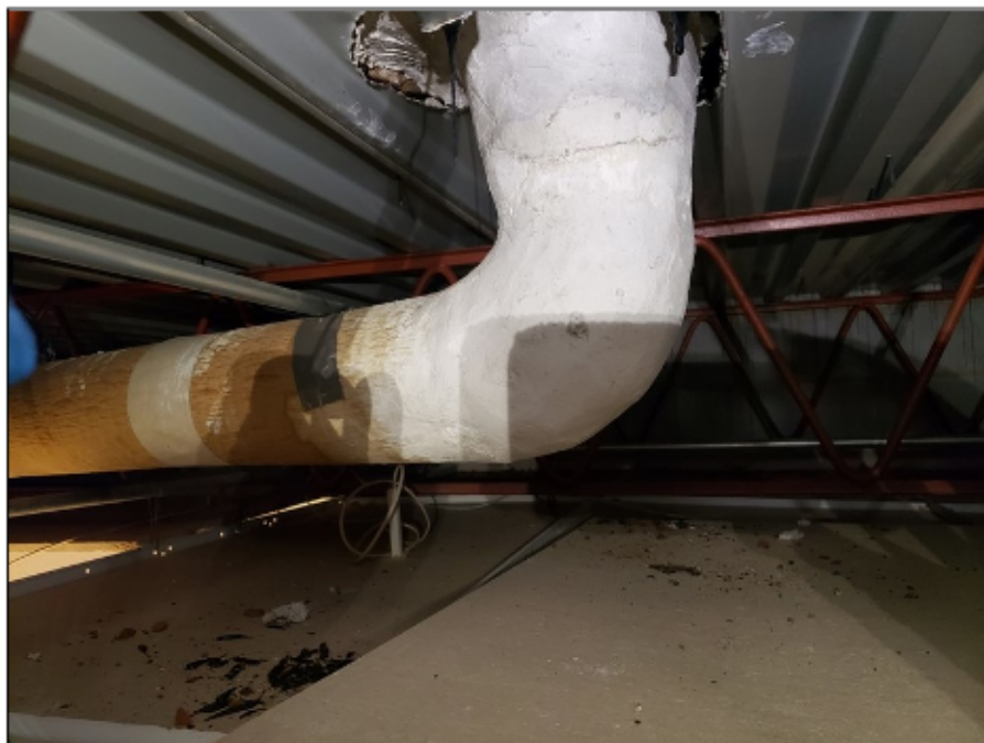
2 - ACM - Mudded Roof Drain Fitting
