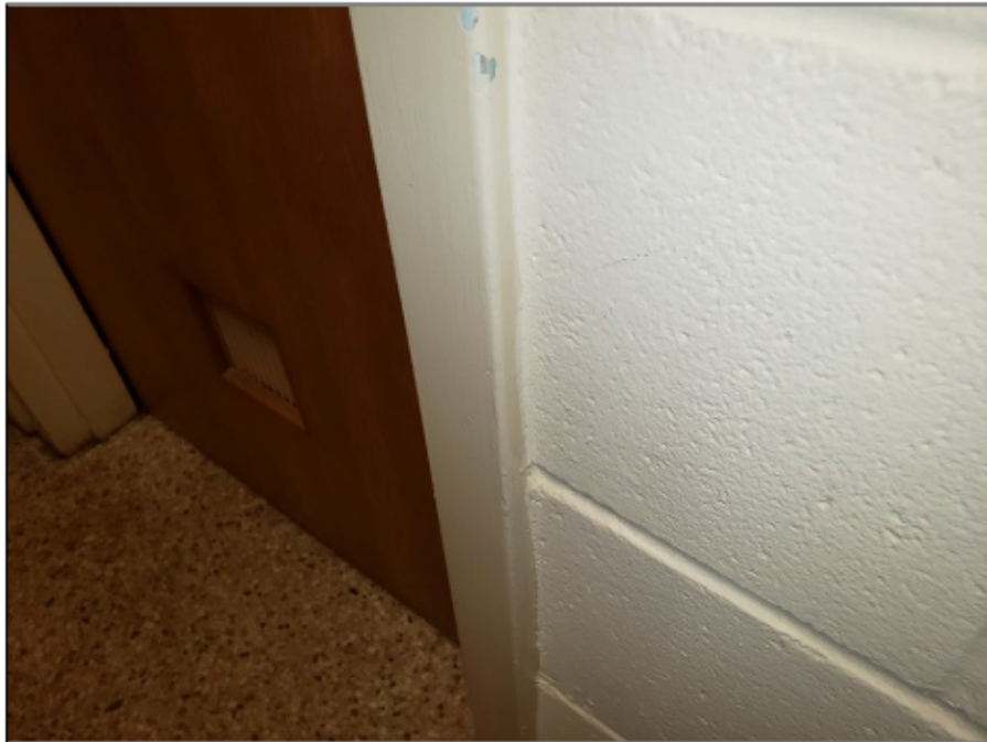
4 - ACM - Door Frame Caulk at CMU Block Walls
